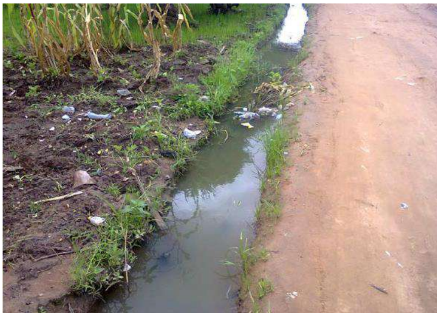
Figure 5. Lack of proper drainage
