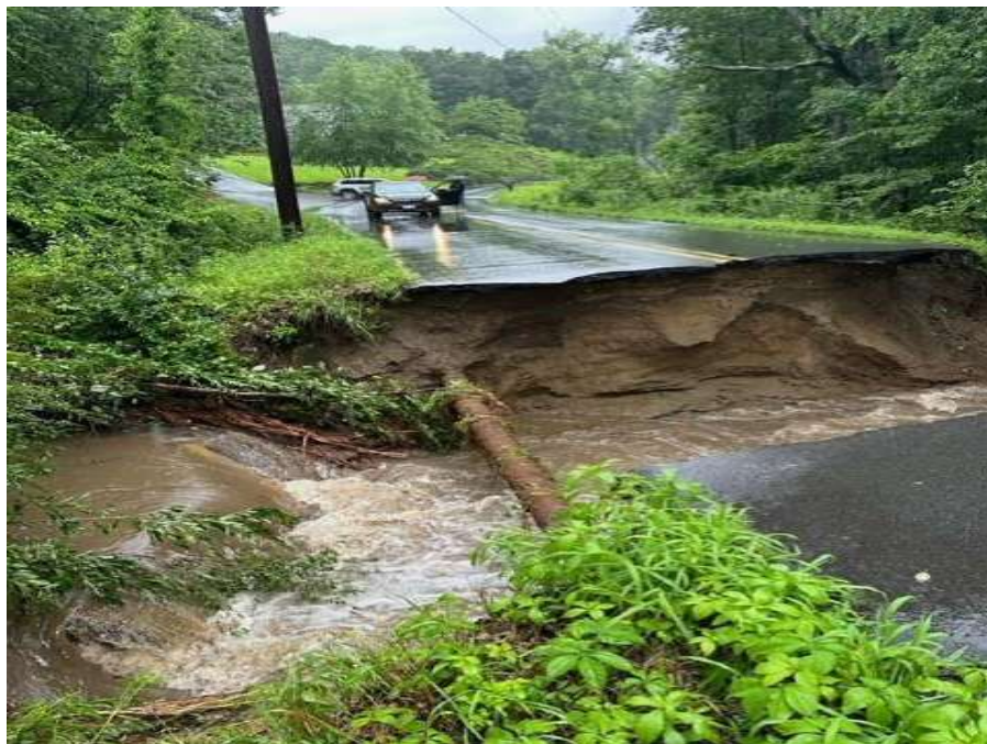
Figure 3. Road cut contributing to flooding hazard.
